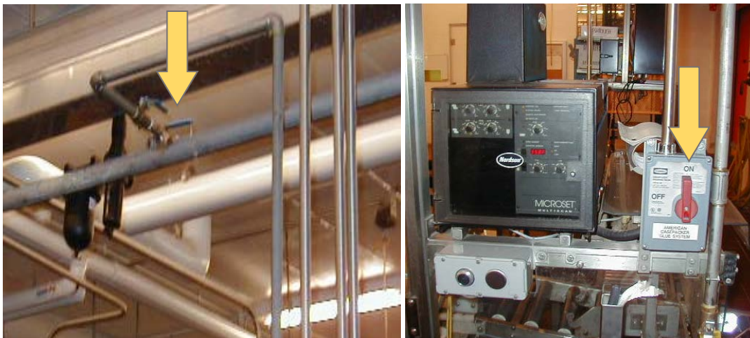
(#1) Compressed air isolation valve
