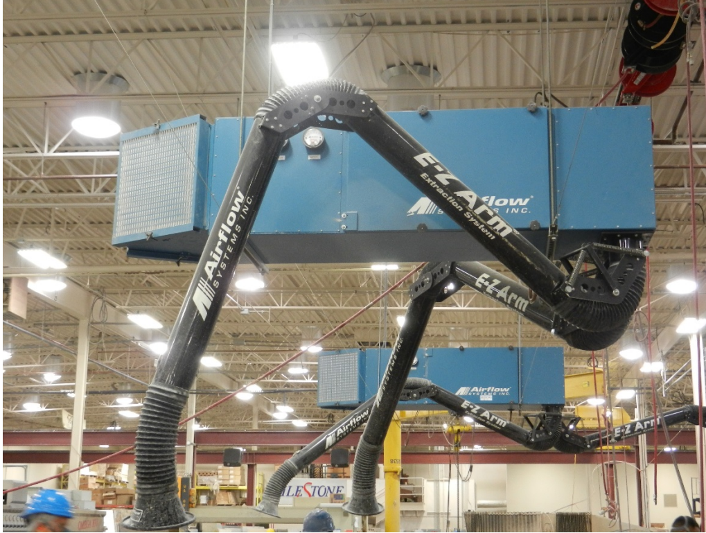
Figure 3. Two air cleaners, each equipped with two E-Z Arm® High Flow Extractors.
