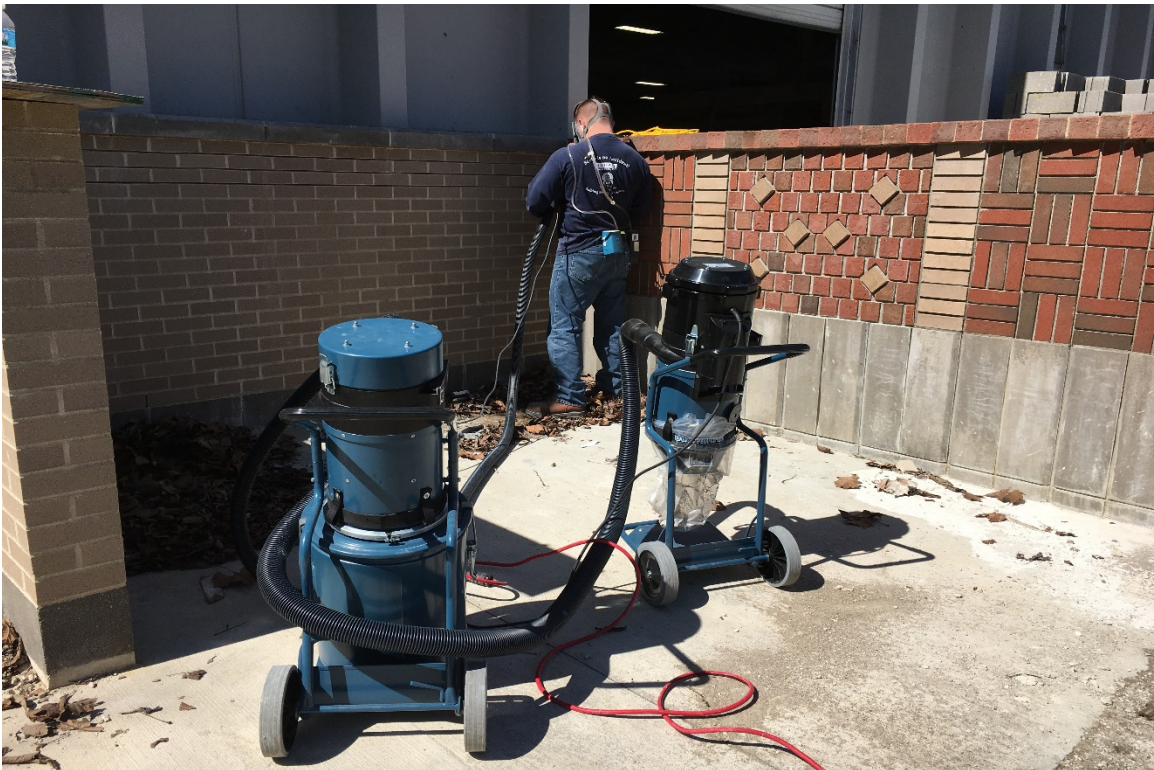
Figure 3 - Pre-separator (left) and vacuum cleaner (NIOSH photo)
