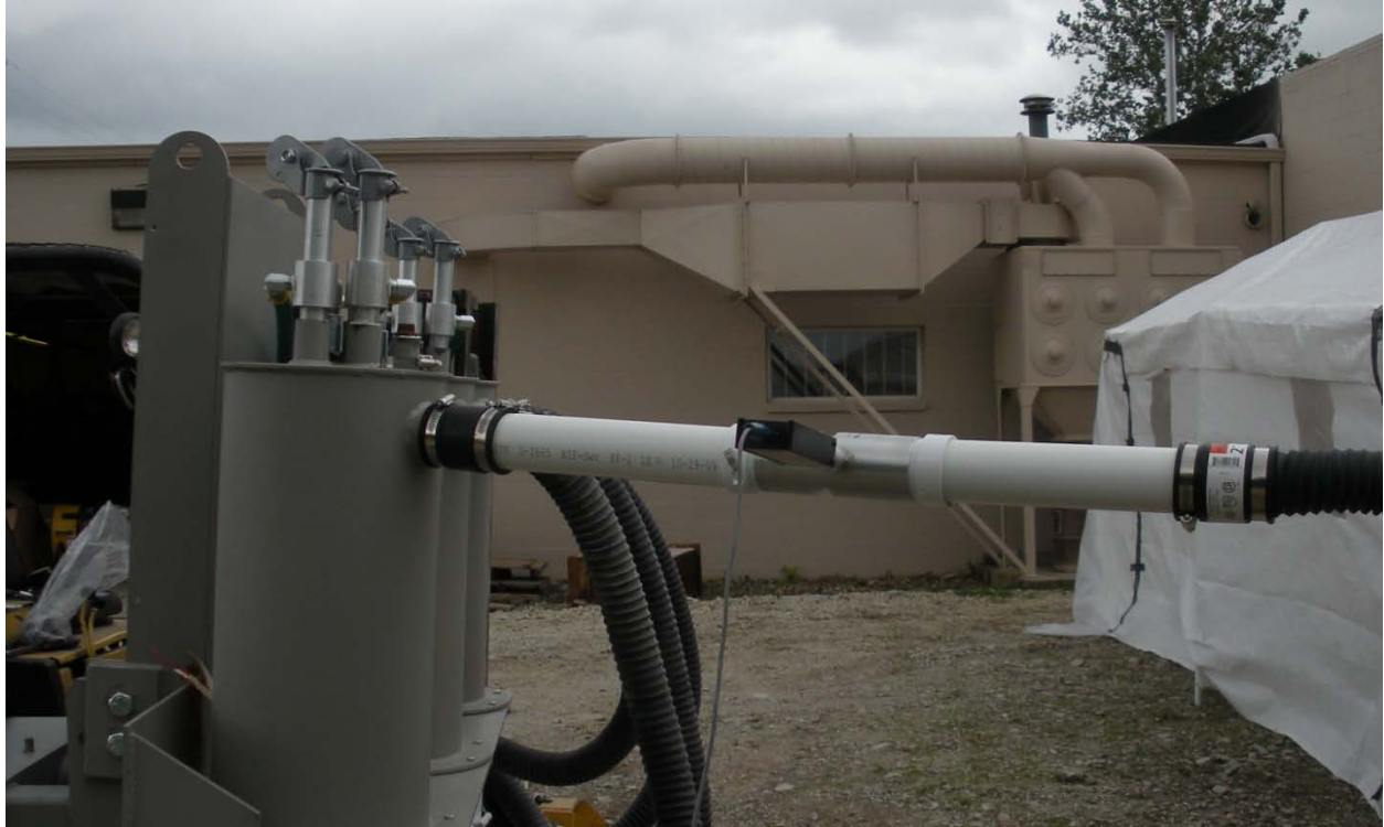
Figure 5 - Exhaust Air Flow was also Measured with the Meter in Line Between the Hood and the Dust Collector
