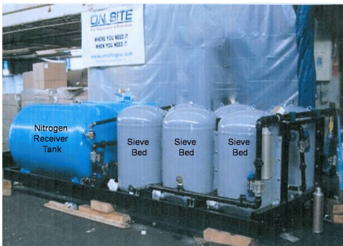
Figure 19. Photograph of On Site Gas Systems in-mine nitrogen gas generation plant (Trevits et al., 2009).
