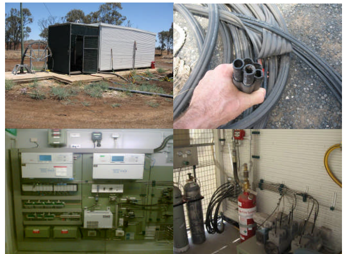
Figure 5. Continuous atmospheric gas monitoring system used in Australia. Top left: Monitoring shed over mine showing borehole and sample tubes. Top right: Close-up of sample tube bundle. Bottom right: Sample tube pumps. Bottom left: Inside monitoring shed showing gas analyzers and controller (Zipf et al., 2007).
