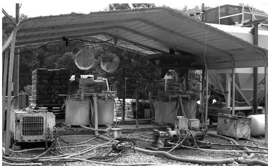
Figure 18 — The two-components (powders) used to produce the CSA grouts are packaged separately in bags and delivered to the pumping site where they are mixed with water.
