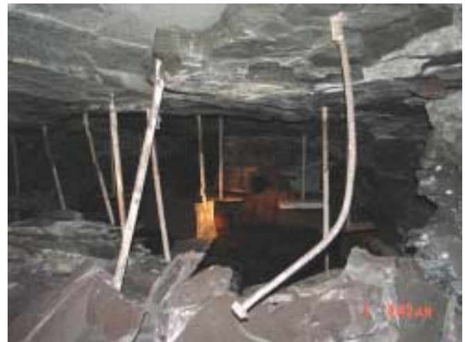
Figure 8. Photograph of roof bolts exposed by weathering of weak shale at Mine B.
