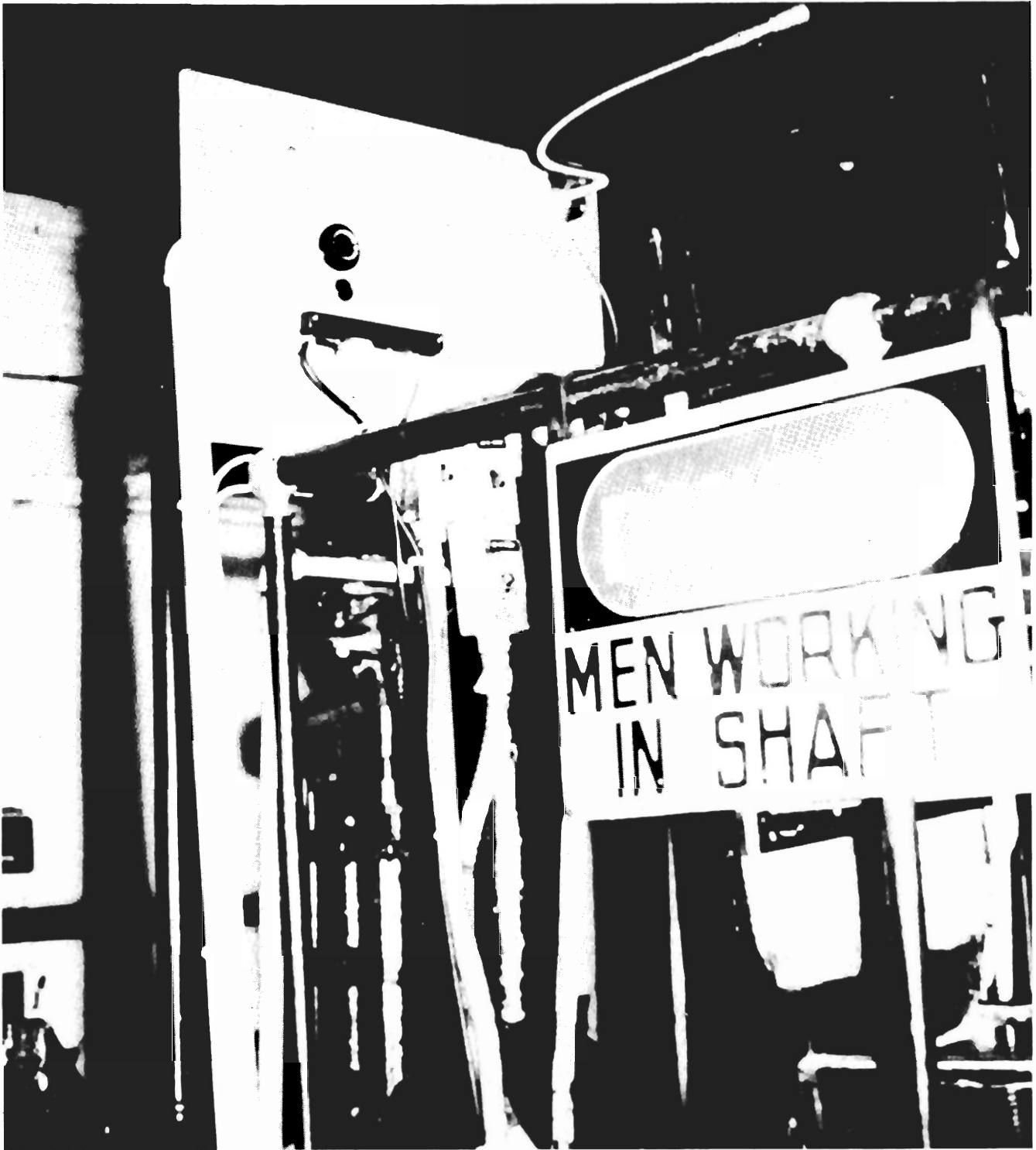
Figure 5-38. Hoist Room Transceiver With Boom Microphone.
