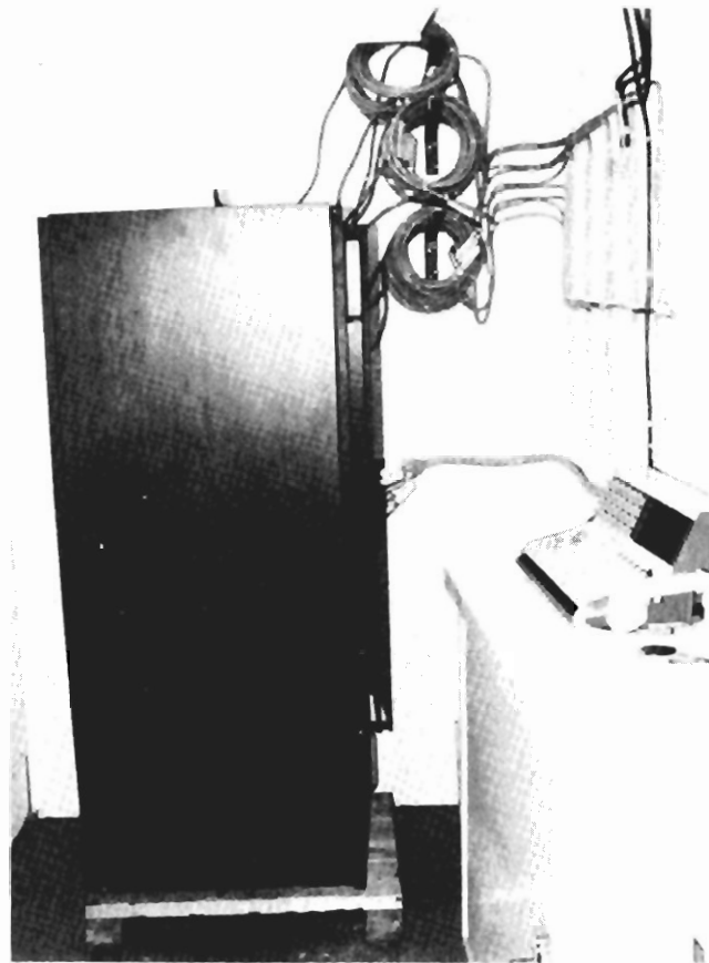
Figure 4-27. Rock Burst Monitor Room PBX Installation.
