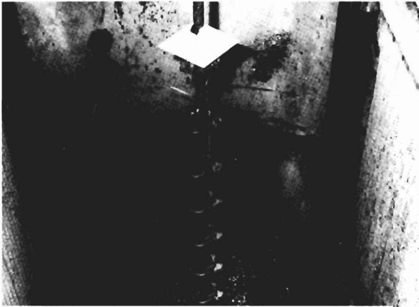
Figure 5-7. Inductive Coupler and Rock Shield Mounted Around the Hoist Cable Above the Man-Cage.
