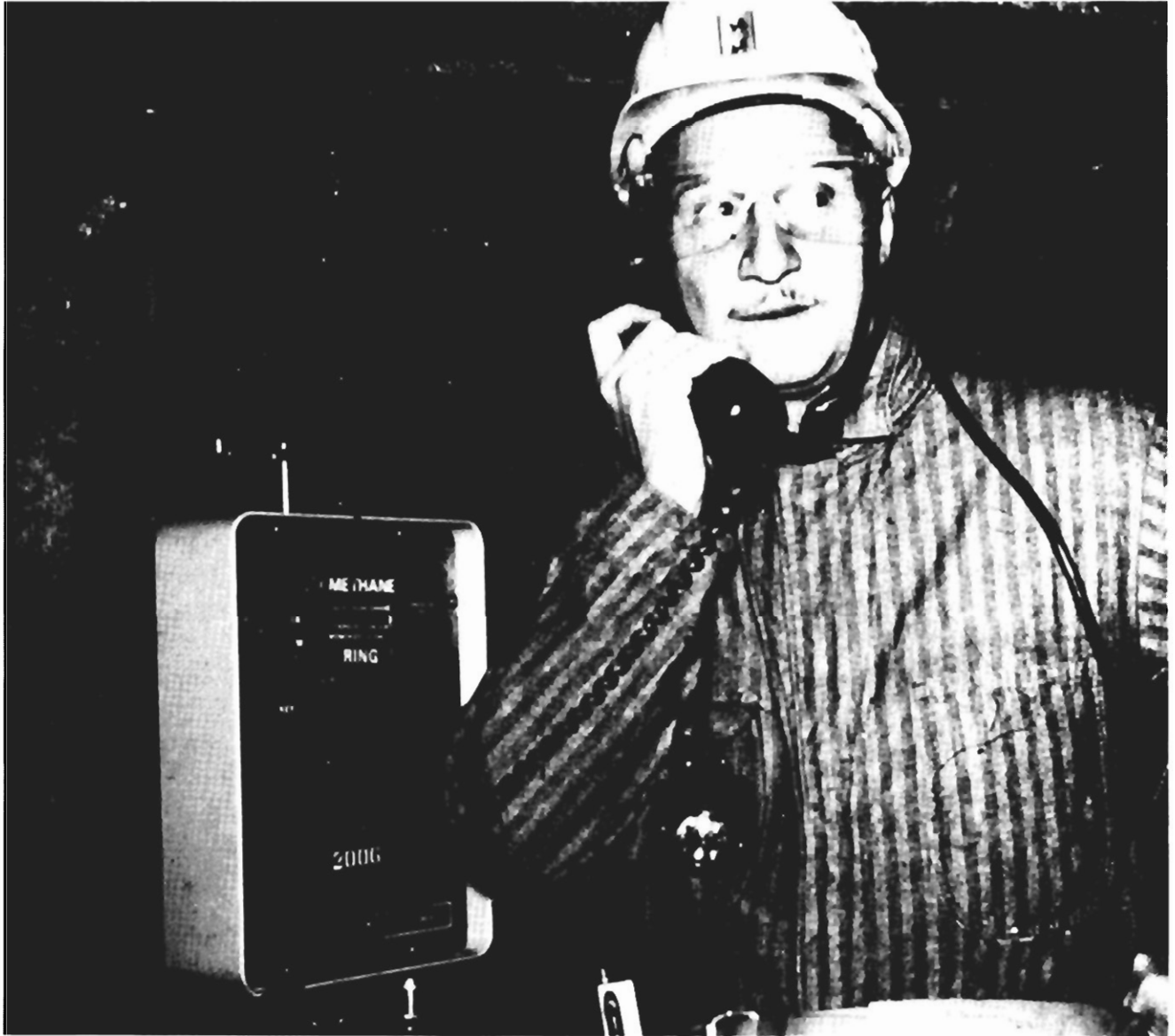
Figure 5-29. Underground Telephone Mounted on Jackpost.
