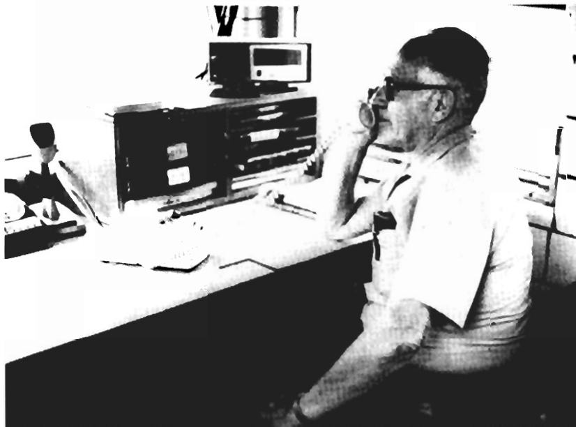
Figure 5-25. Intercom Telephone in Surface Guardhouse.
