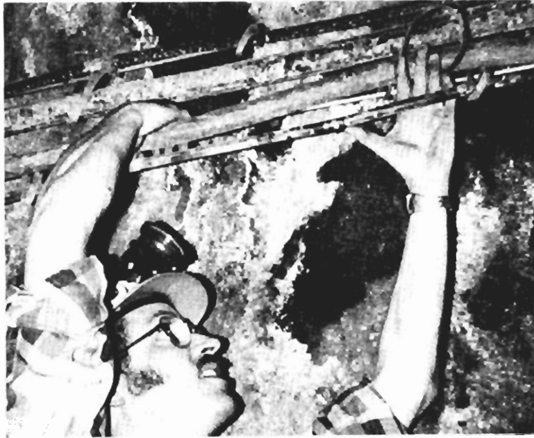
Figure 3.8. Blasting Damage Done to Unprotected Radiax in Loading Drifts.
