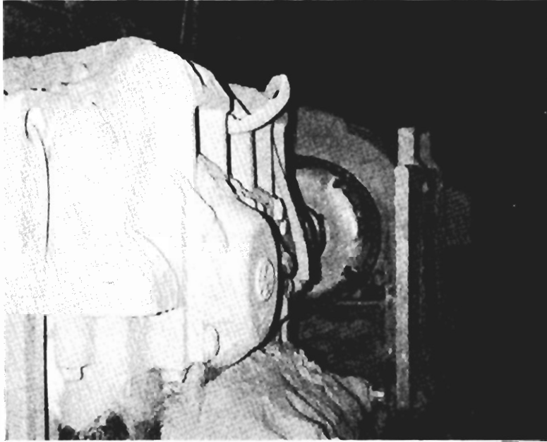
Figure 3.16. Ore Haulage Belt and Drive Motors.
