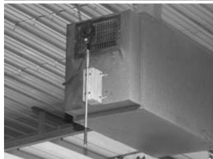
Figure 5. Location of gravimetric samplers at the intake side and the recording vane anemometer at the louver exhaust side.
