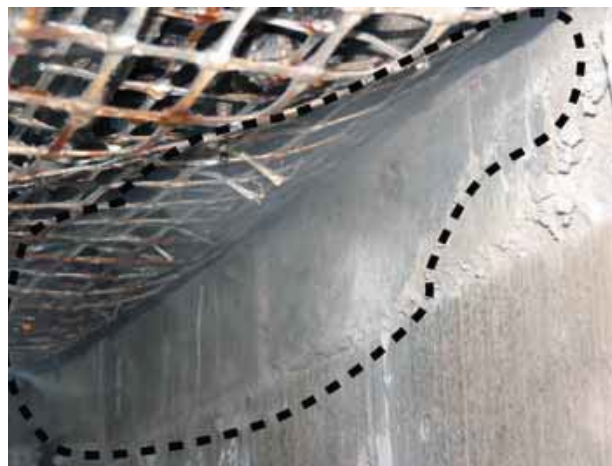
Figure 3. Smoke leaking through the stopping perimeter at the roof for Test 2
