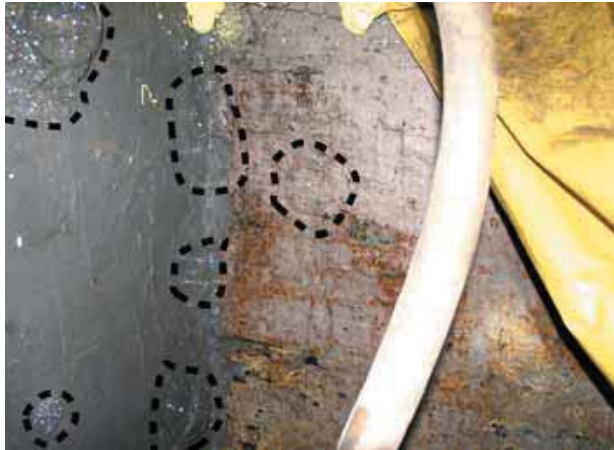
Figure 6. Soap bubbles on stopping and at the right rib at 1245 Pa (4.5 in) WG
