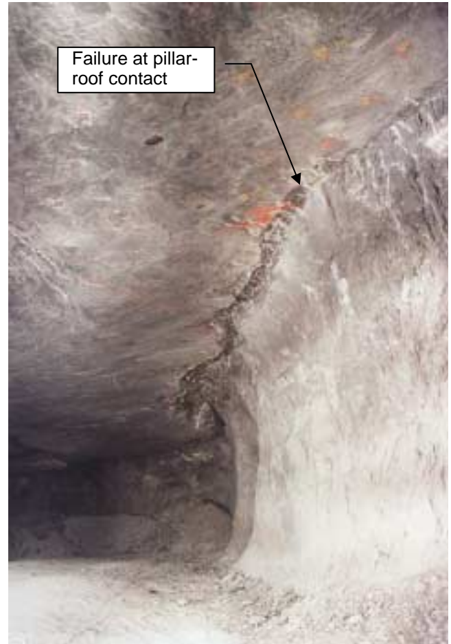
Figure 1. Photograph showing failure at pillar-roof contact after loose rock has been removed and roof has been re-supported.
