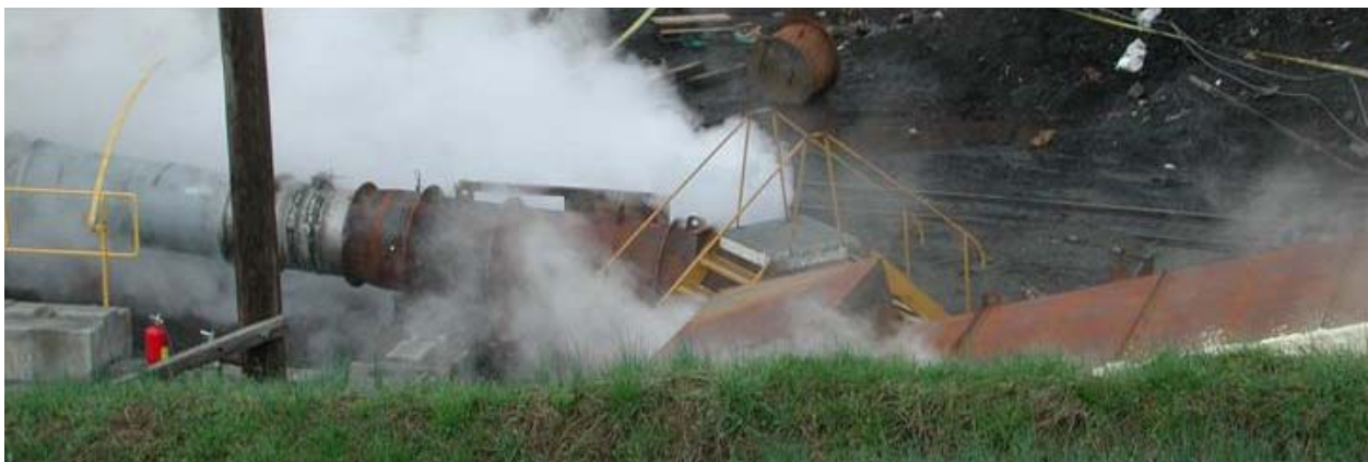
Figure 4. GAG 3A jet engine system interface with Sugar Run Slope. Note steam indicating exhaust gas leakage.
