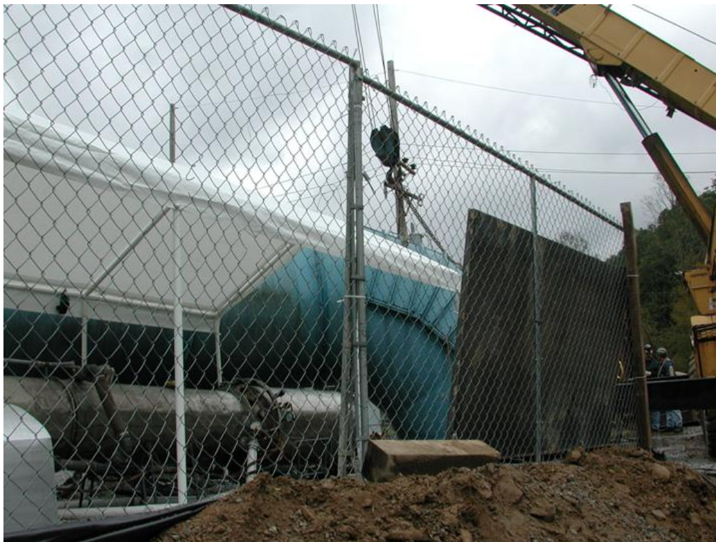
Figure 10. Photo of GAG 3A System set-up at 8A Bleeder Shaft, Pinnacle Mine. Note fabricated shaft hood for docking.
