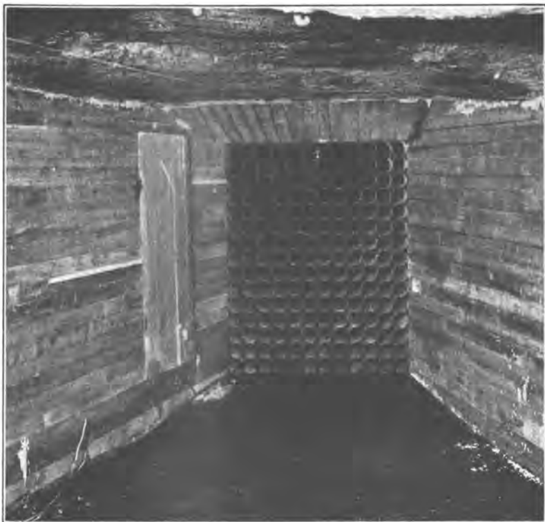
FIGURE 8.—Approach side of 1B-100 air-measuring station
