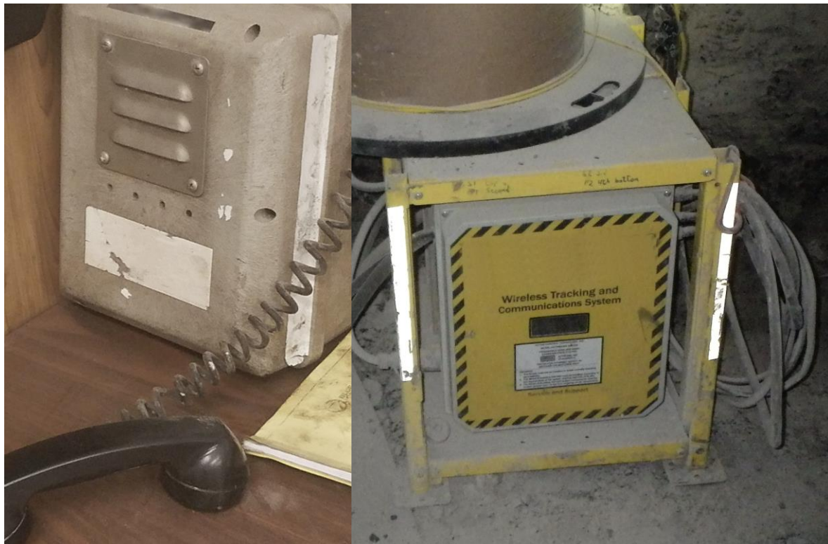
Figure 17. Surface mine phone (left) and underground wireless tracking and communication systems (right).
