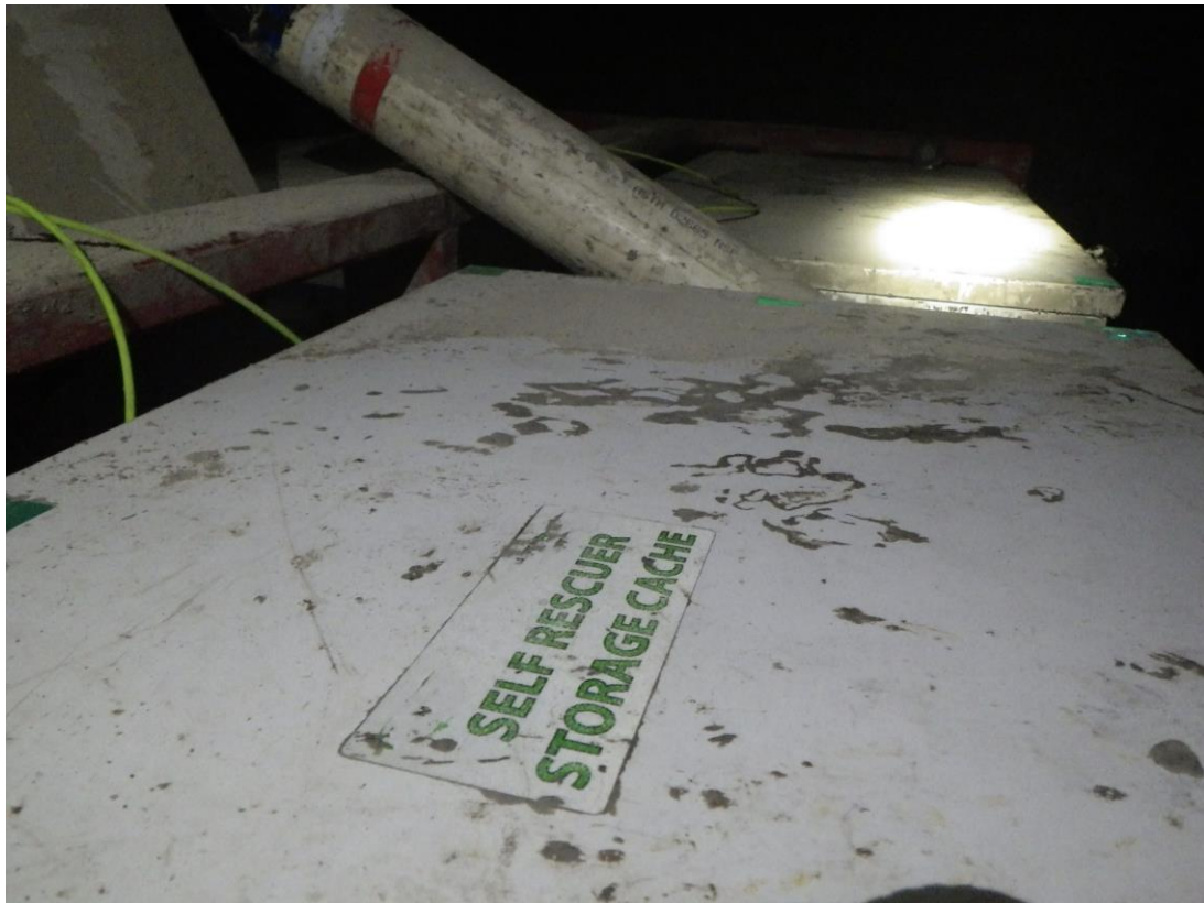
Figure 6. Tagline/tetherline and escapeway map situated at an SCSR cache location.
