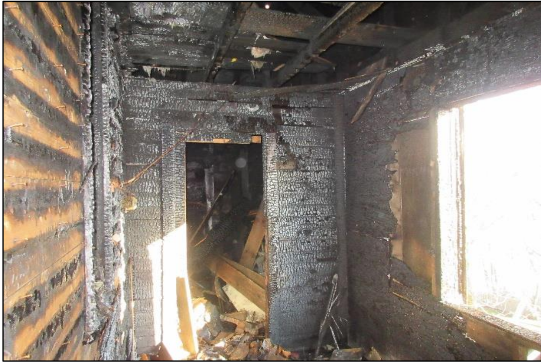
Third floor porch shed breached by Rescue 2 where Ladder 5 Lieutenant took shelter. (NIOSH Photo)
