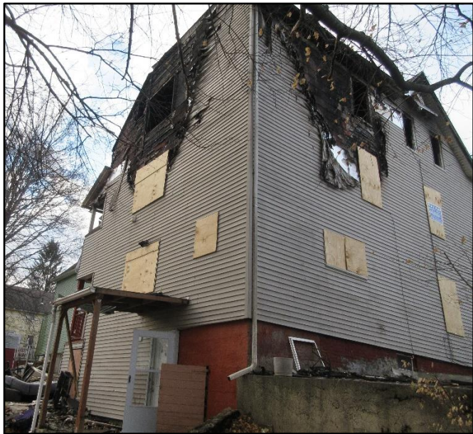
Side Bravo and Side Charlie of the structure. (NIOSH Photo)
