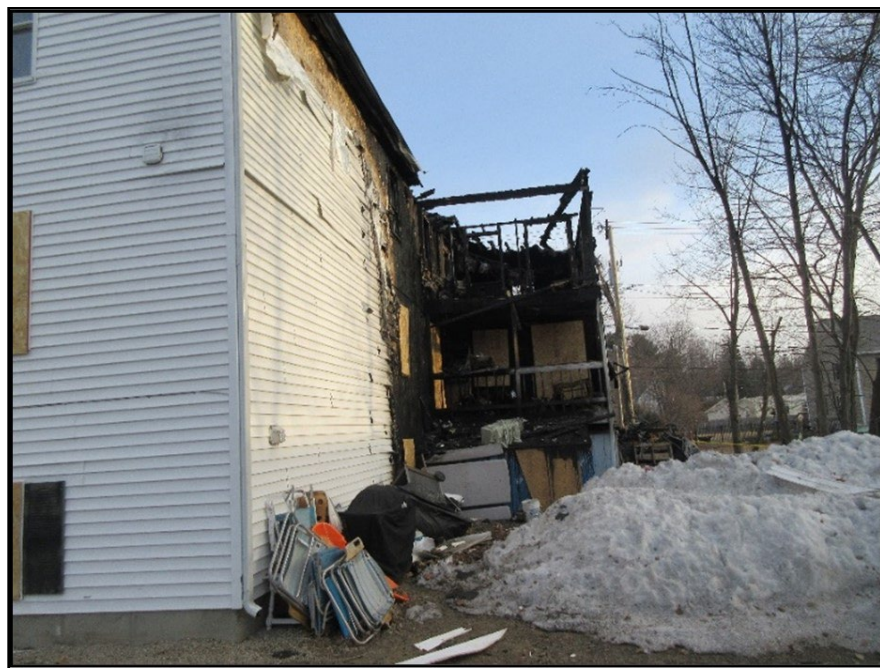
The Side Charlie 3 rd floor porch where the captain and firefighter 1 were removed. (NIOSH Photo)
