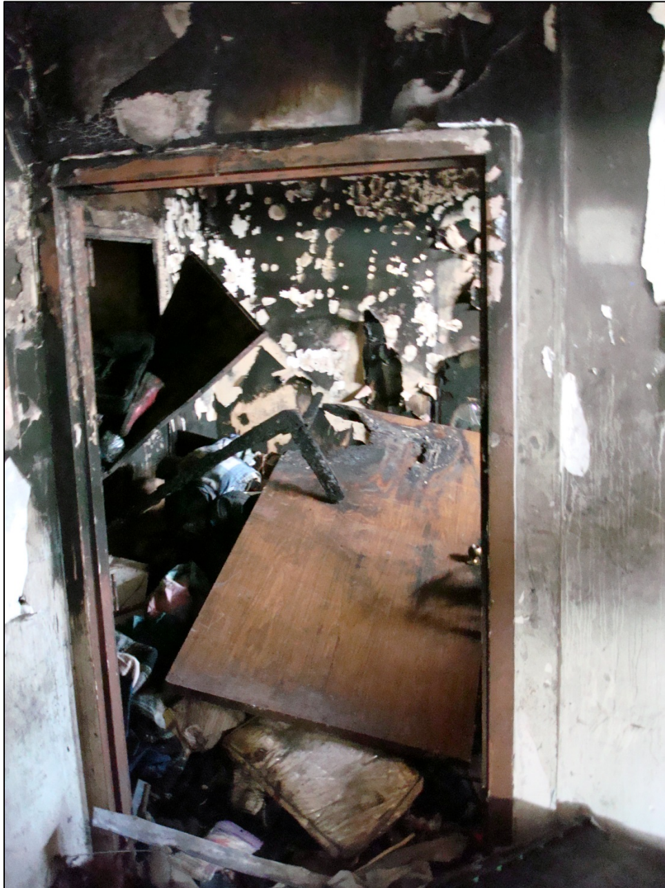
Photo 3. View is from living room looking into bedroom. Note that the door was removed during the recovery operation. (NIOSH photo.)
