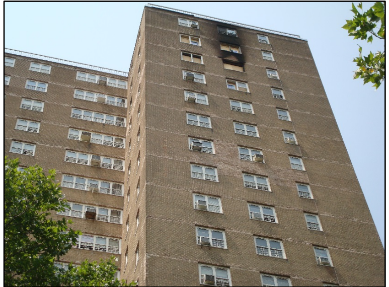
View of apartment building looking up from street level. Center window is room of origin.
