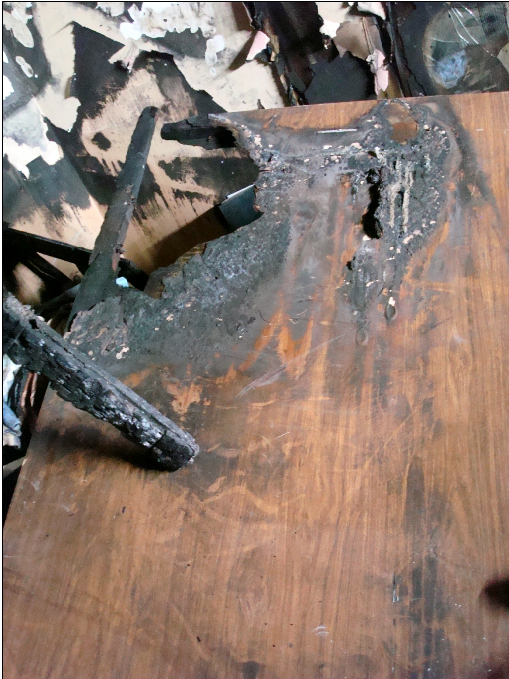
Photo 4. Close-up view of bedroom door. Note the burn-through at top of door. It is believed that the door burned through allowing fire to extend from the bedroom. (NIOSH photo.)
