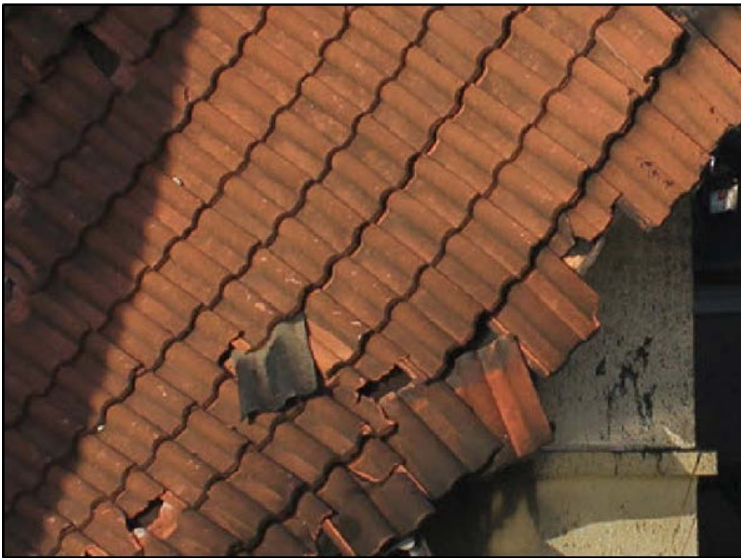
Photo 2. Concrete Roofing Tiles - Post Fire (NIOSH Photograph)
