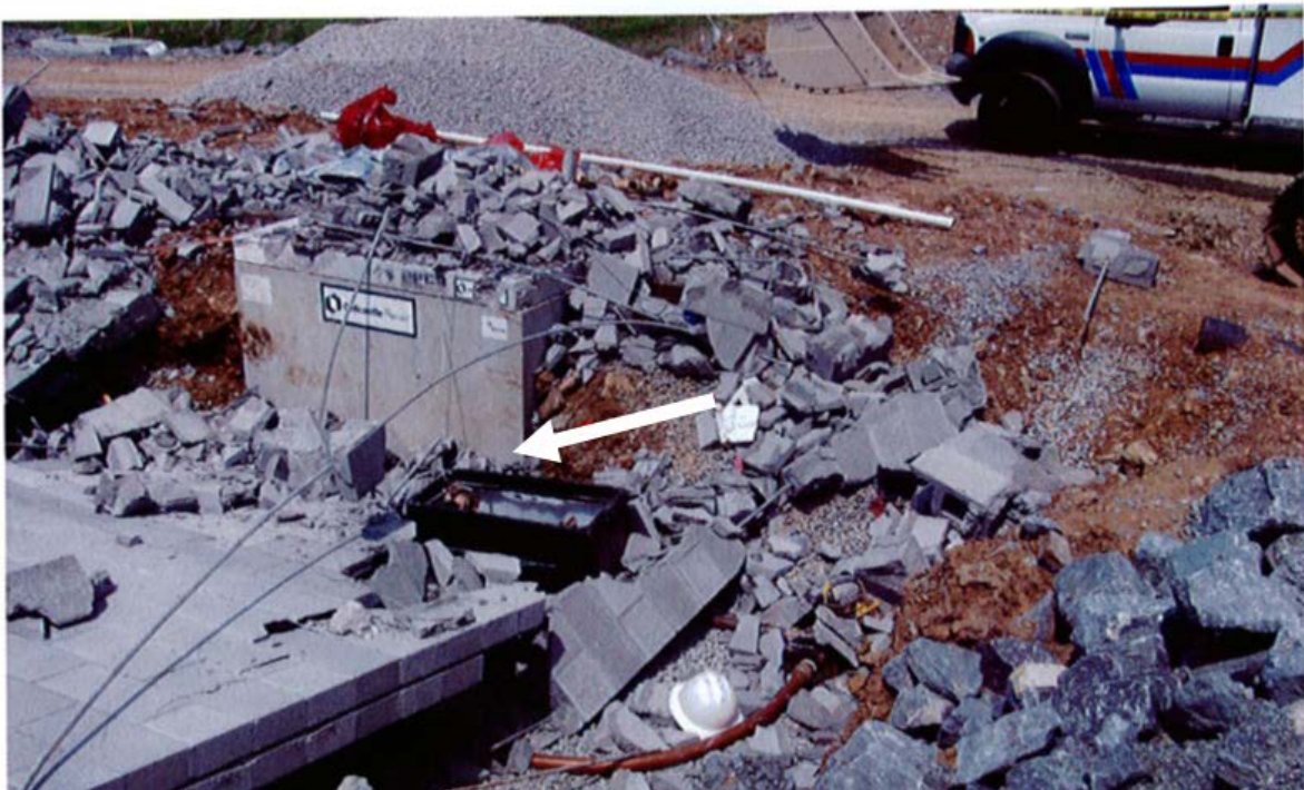
Photo 4. Concrete meter box. Arrow indicates where three excavation employees were working. (Photo courtesy of TOSHA.)
