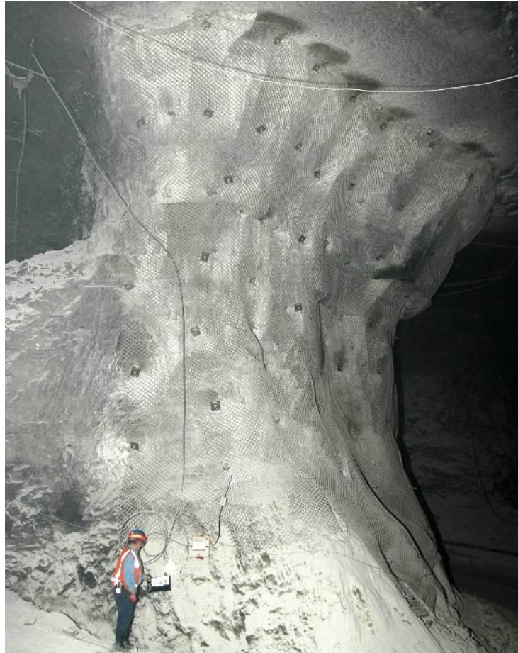
Figure 9. Pillar that has been clad with chain link mesh to prevent further deterioration of the ribs.
