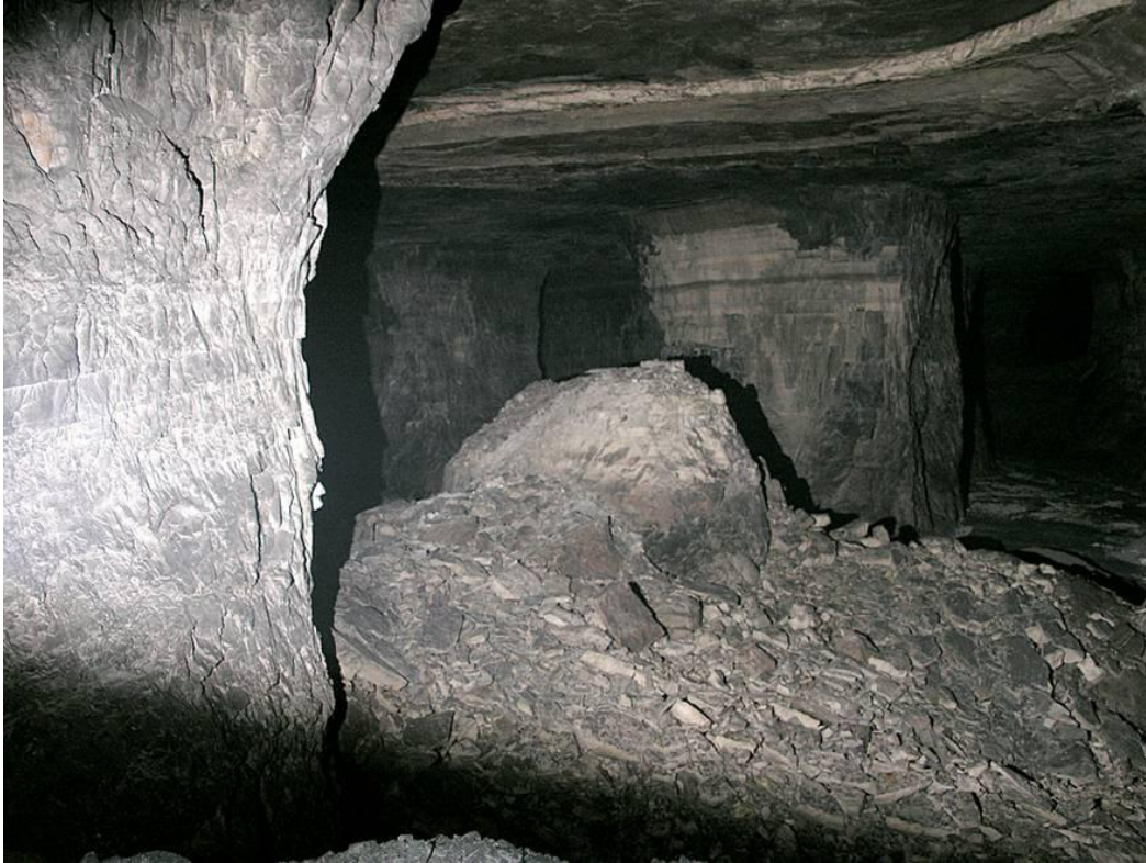
Figure 6. Remaining stump of a collapsed pillar in an abandoned area. Thin, weak beds in the pillar and moist conditions are thought to have contributed to the failure. The width-to-height ratio was 0.82 and average pillar stress about 11% of the UCS.
