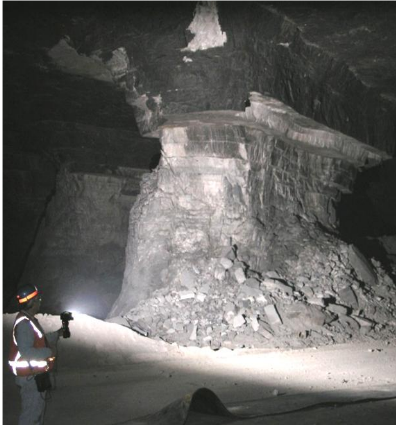
Figure 17. Pillar damage observed in rock containing thin, weak bands. Note spalling of the intact rock material between the weak bands.
