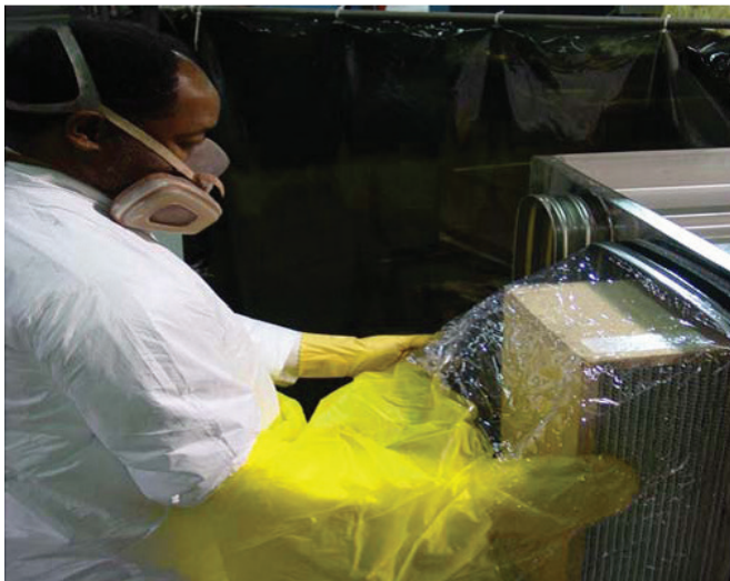
Figure 19. Removal of a dirty air filter from a ventilation unit into a plastic bag to minimize worker exposure to particles captured by the filter unit (Used with permission from Filtration Group Inc. [2012])
