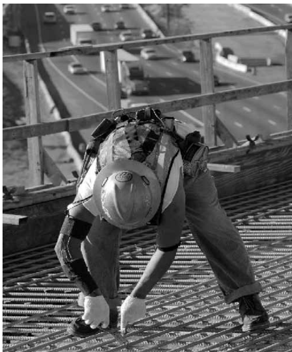
Figure 1. Rebar tying using pliers. Note the bent posture and awkward hand position.
