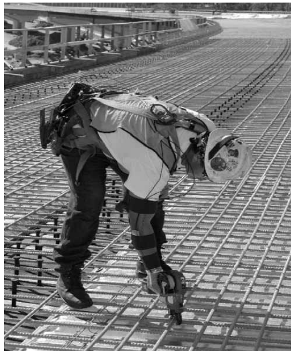
Figure 2. Rebar tying using a MAX-USA RB-392 power tool. Note the bent posture.
