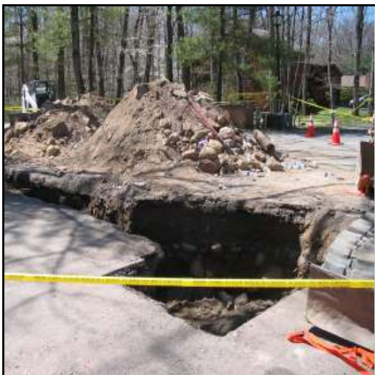
Figure 3: Location of collapse. Note spoils piles and equipment located less than 2 feet from the edge of the trench (courtesy of OSHA)
