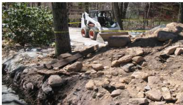
Figure 2: View of the west wall of the excavation south of the "T." Note the boulders and loose rock/dirt on the excavation face as well as the location of the spoils pile within 2 feet of the edge of the trench. (courtesy of OSHA)
