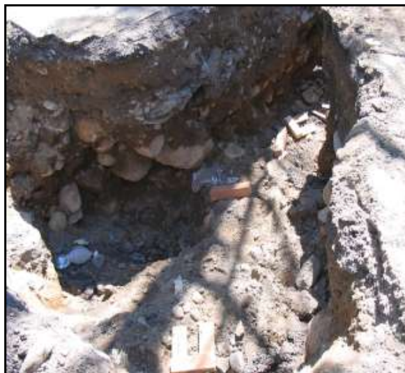
Figure 4: Area of trench collapse Note the large boulders hanging from the excavation faces and undermined areas on the edge of the trench (courtesy of OSHA)
