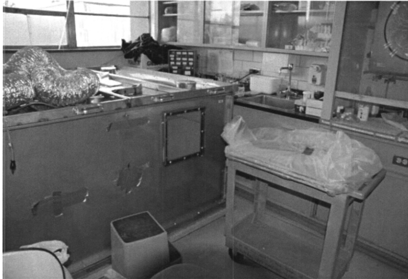
Figure 3. Drywall being removed for transportation to an area to be sampled and treated.
