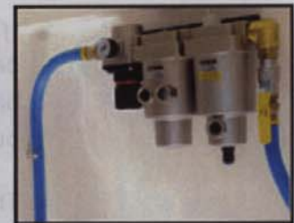
Mine Air Filter System
